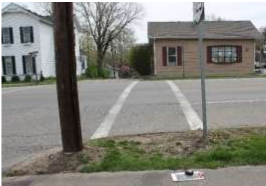
Figure 2.4 Crosswalk lacking signage and a curb ramp at West and Franklin
